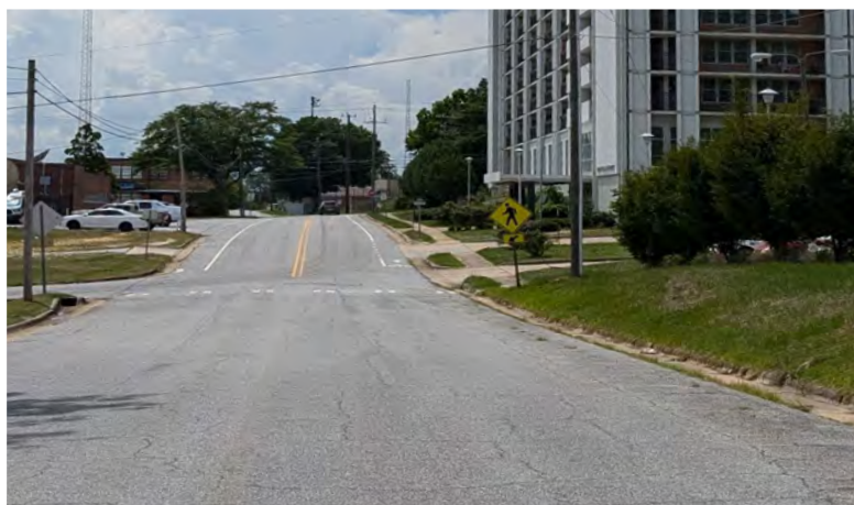
Sidewalk facilities on one side of the street end abruptly.
